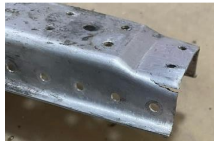
Cracked stringer after it was removed
